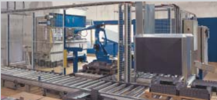
The large conveyor has room for six filled Euro-pallets without collar. Infeed magazine for 15 empty pallets.
